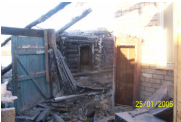
Aftermath of the fire
